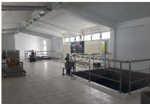
Figure 7. Coagulation and flocculation facility
