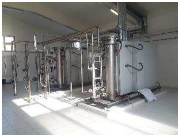
Figure 8: Ozonation facility – ozone generators
