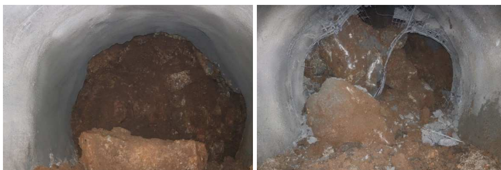
Figure 21. Falling of large blocks from the fault zone during the construction of the tunnel at chain. km 1+839
