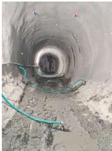
Fig. 5. Radially arranged drainage measures in the pilot tunnel (Source: IGT Geotechnik und Tunnelbau).
