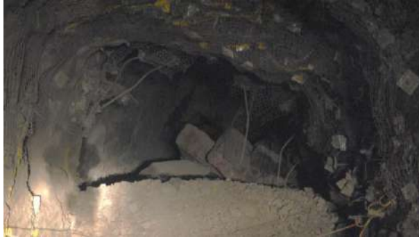
Fig. 6. Blocky metasandstone on extraction level. Block falls observed from hanging wall of unsupported stope.
