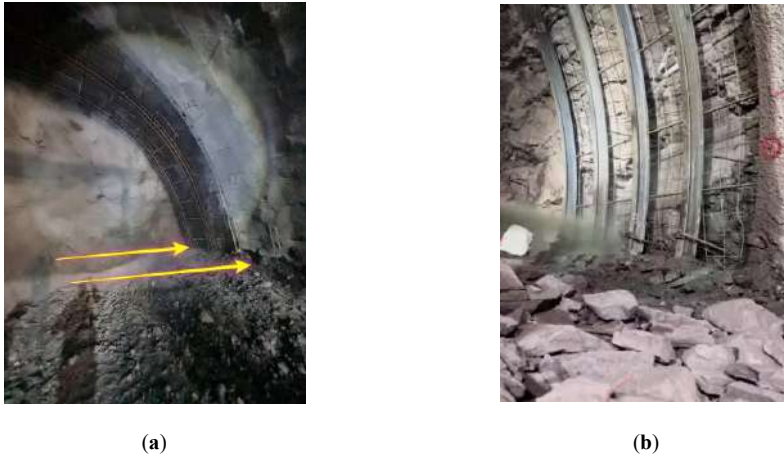
Fig. 2. (a) Primary support without anchors and propiate temporary foundations; (b) Installing multiple steel ribs in the stable ground with no stiff support on the ground.
