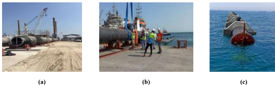
Fig. 14. Onshore fabrication works. (a) Milaha Port site; (b) HDPE pipework being assembled; (c) HDPE pipework transition.
