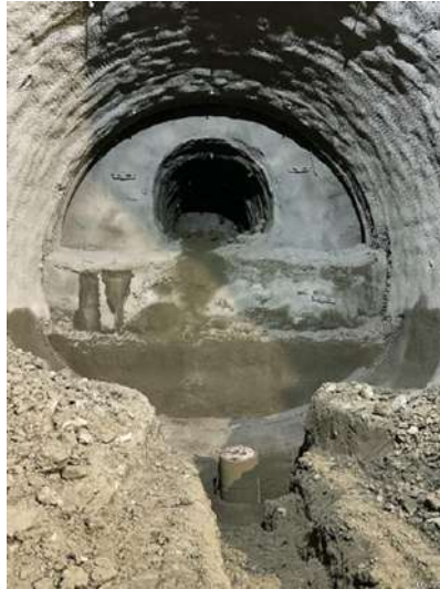
Fig. 4. Pilot tunnel within the excavation profile of the station tunnel (Source: IGT Geotechnik und Tunnelbau).
