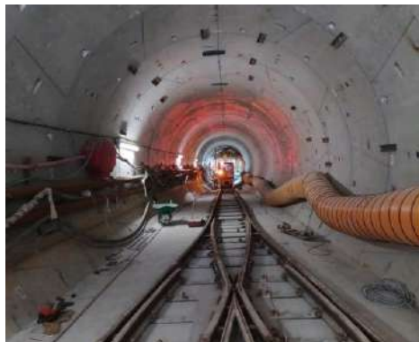
Fig 13. Installation of California switches and final arrangement for TBM regular mining activities.
