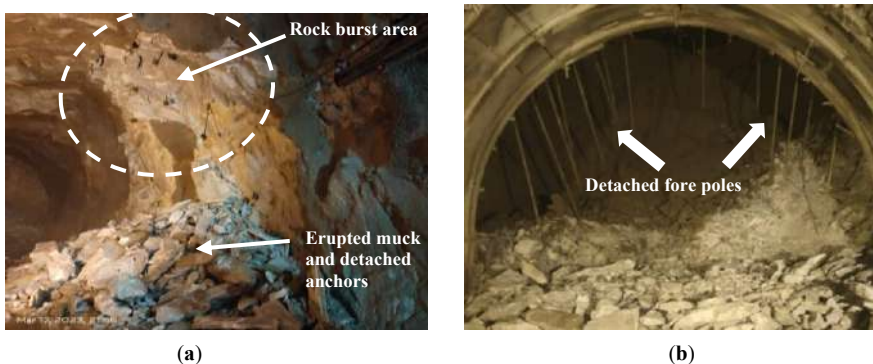
Fig. 9. (a) Rock spalling resulted in detachment of shotcrete and rock anchors around RD \pm 5284 m; (b) Fore poles detached and hanged after multiple episodes of rock bursts at the face and crown around RD \pm 5352 m.
