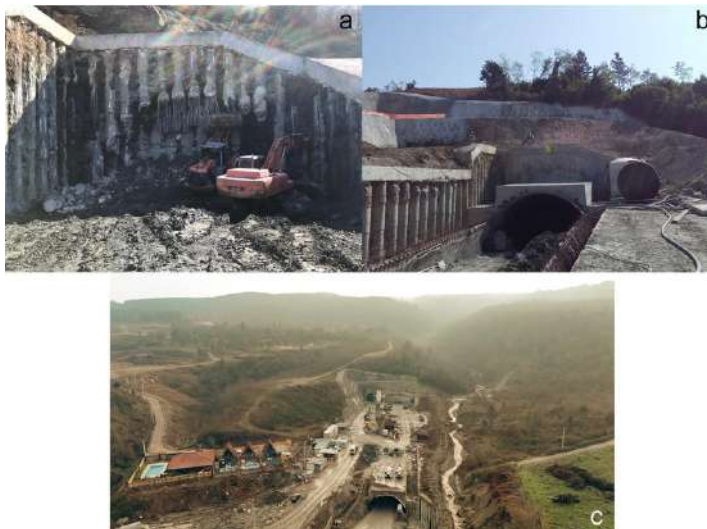
Fig. 12. T1 Tunnel portal construction stages (a: completion of bored pile construction, b: cut-and - cover construction and backfilling stage, c: T1 Tunnel portal completed status).
