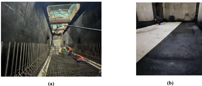
Fig. 5. General view of the work during the installation of sprayed waterproofing with double-sided adhesion: (a) installation of a metal frame on waterproofing laid on diaphragm walls and on concrete preparation, before concreting wall structures without hollows for backfilling the soil and a tray plate; (b) installation on a primed
