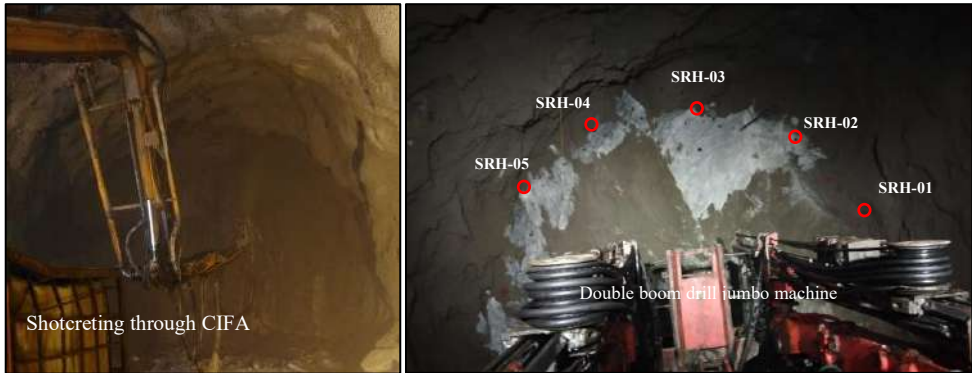
Fig. 10. (a) Application of normal shotcrete and SFERS layer-wise on tunnel face, crown, and side walls; (b) Drilling of stress relief holes (SRH) at the face using a double boom drill jumbo.
