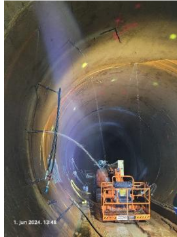
Fig. 15. Installed packers in the right side of the tunnel cross-section at chainage km 7+942.
