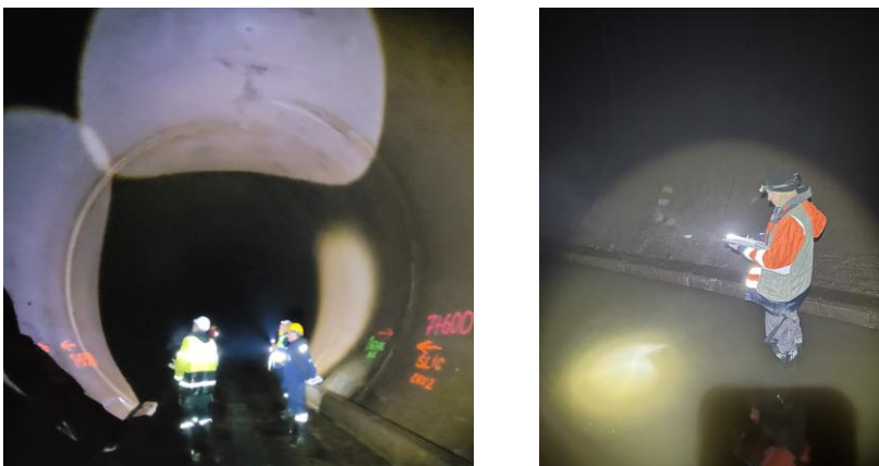
Fig. 3. Visual Inspection – Mapping of Changes in Concrete Lining.
