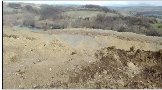
Figure 1 Landslide on the "Landfill 3"
