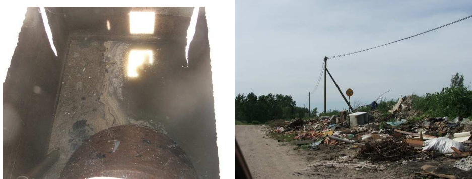
Figure 2. Existing outlet manhole of the sewerage pumping station (left); illegal landfill within the defined sanitary protection zone of the "Petrovaradinska ada" source in Novi Sad [14] (right)
